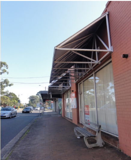
Existing poor amenity and inactive frontage
