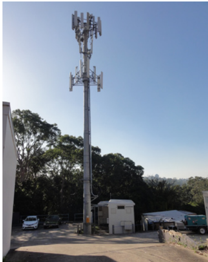
Telecommunication tower and station on site
